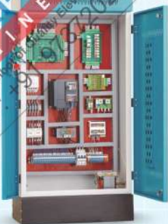
Microprocessor Control Panel
